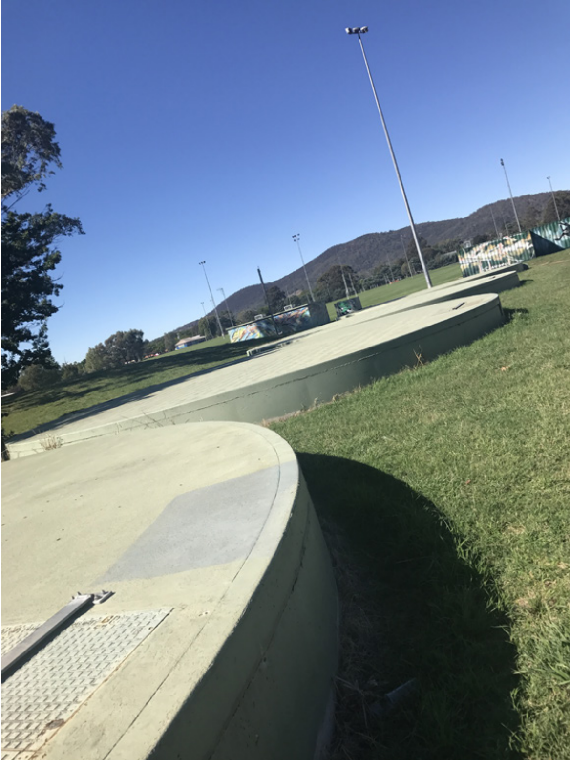
Typical stormwater harvesting tank at Dickson
