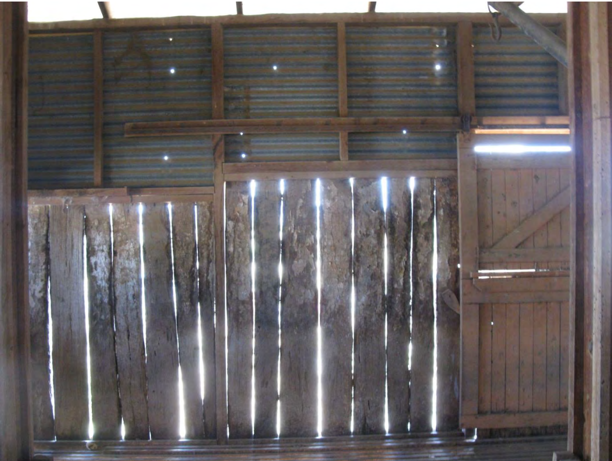
Plate 7. Inside of south wall showing different height slabs and framing for upper corrugated iron clad wall.
