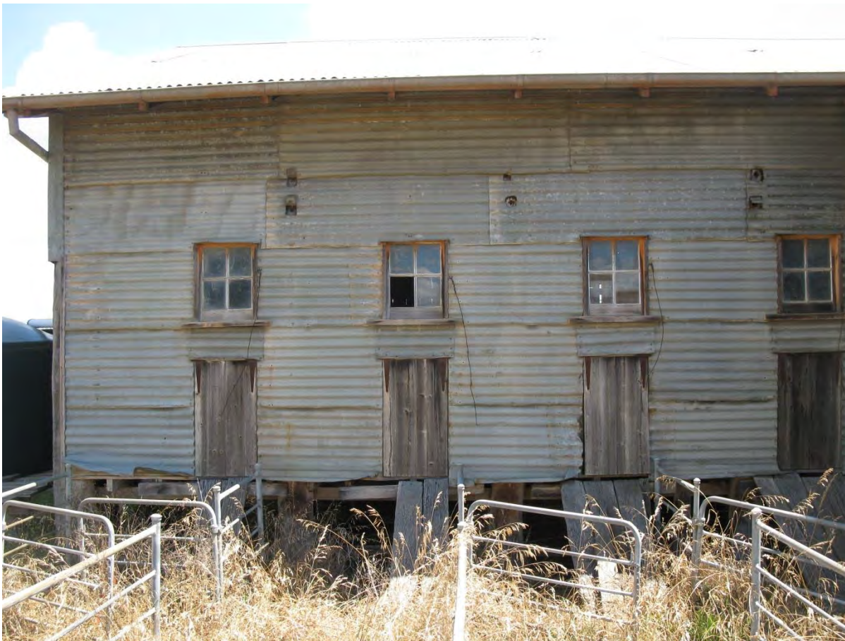
Plate 3. Part north elevation showing sheep chutes – note holes for lineshafting above and right of windows
