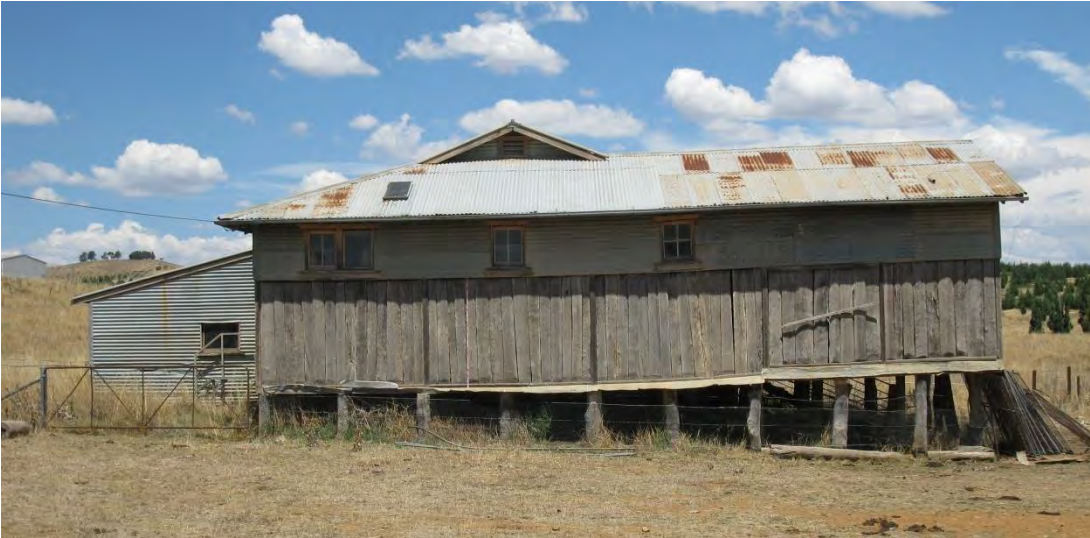
Plate 1. West elevation of shed. Note collapsed and sunken stumps
