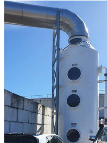
Example odour control system (humidifier) upstream of biofilter
