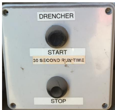
Figure 4: Water Cannon Manual Control Panel
