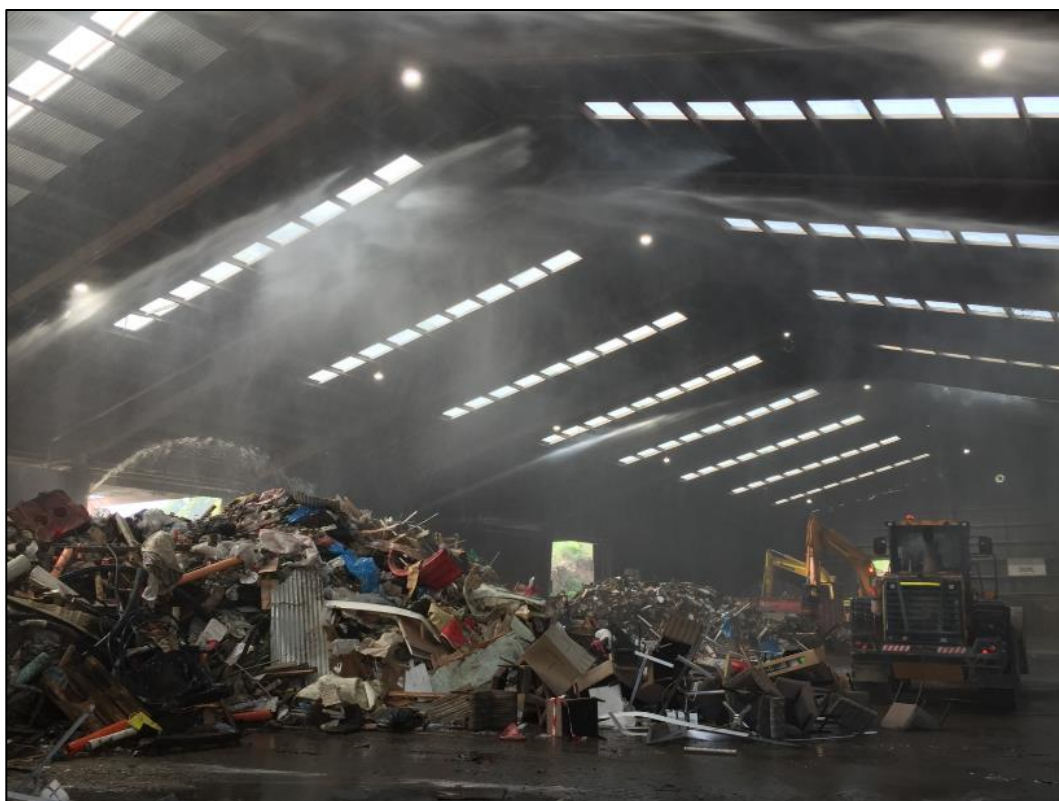
Figure 5: Water Cannons Operational
