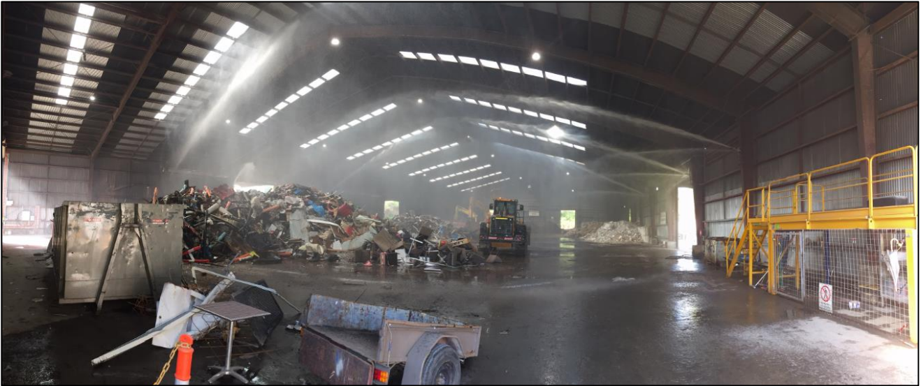
Figure 6: Water Cannons Operational
