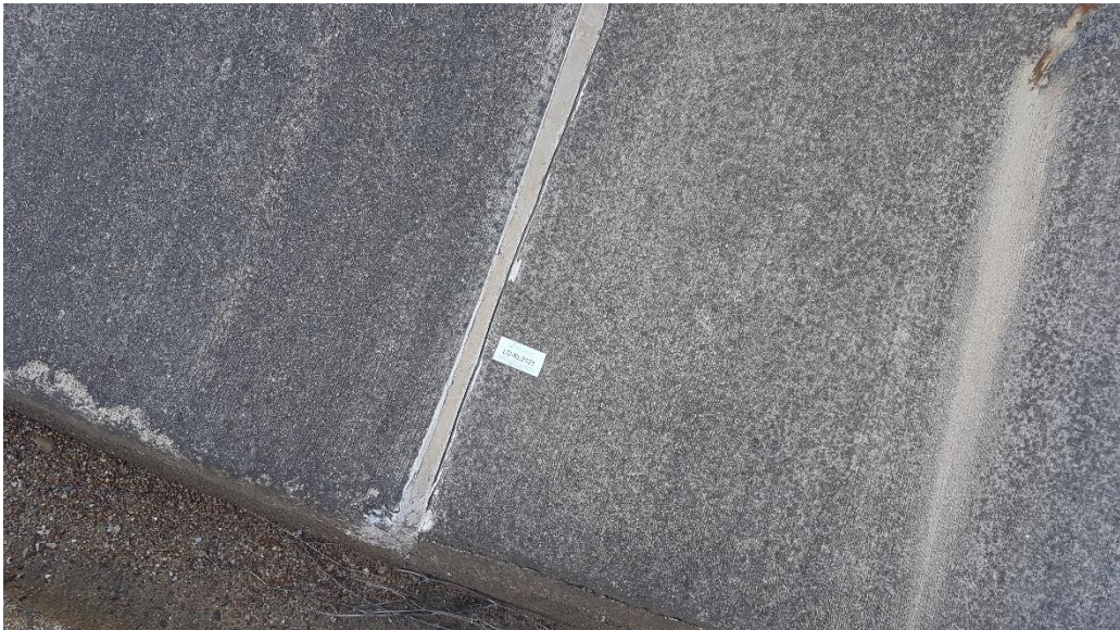
Photograph NA4 Expansion joints to fuel tank concrete pads
