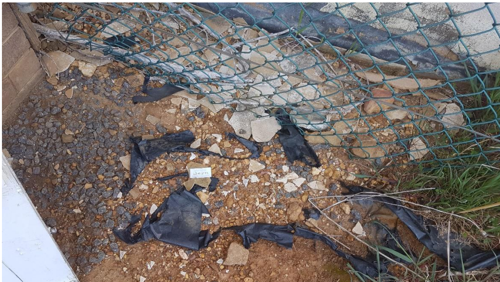
Photograph A2 Around store office External sheet debris (mixed with non-asbestos material)
