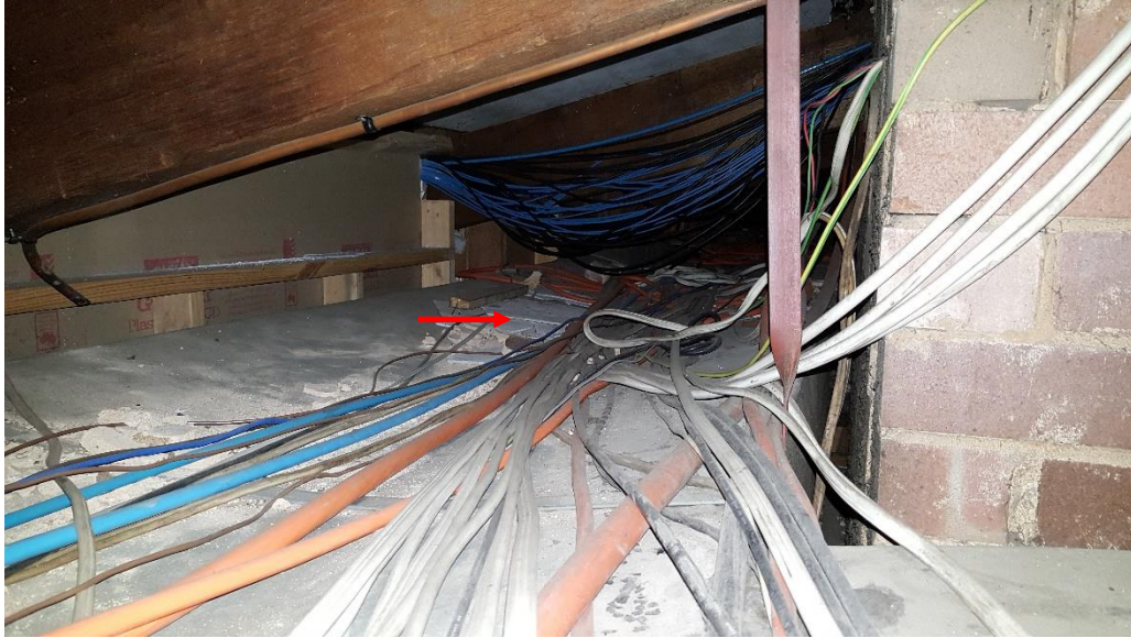
Photograph A9 Main Office Sheet debris to ceiling void
