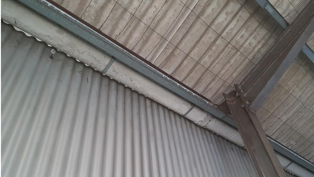
Photograph A7 Store shed (front) Guttering to roof
