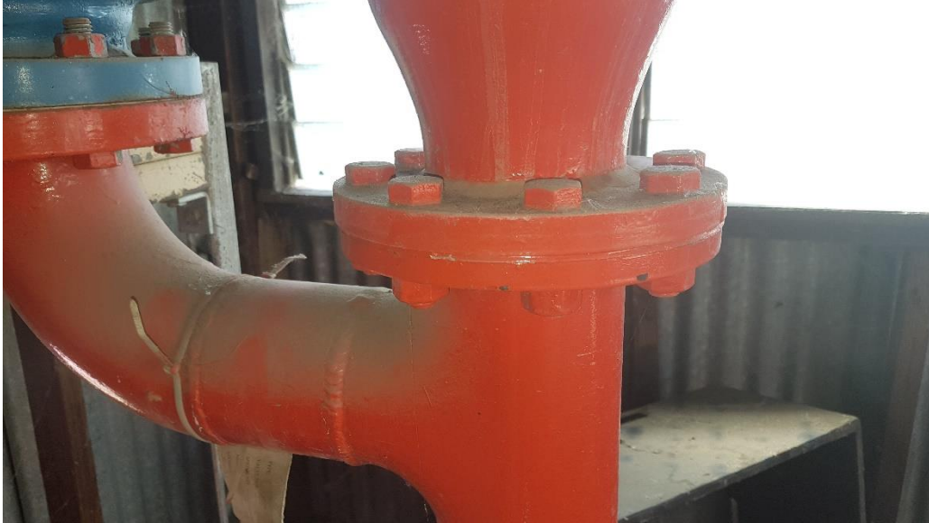
Photograph A3 Fire pump shed Pipe flange joints
