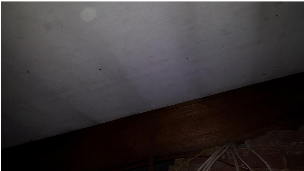
Photograph A8 Main Office Sheet lining to ceiling void
