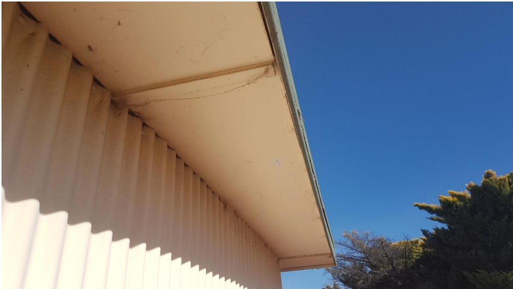
Photograph A4 Fire pump shed Eave sheets
