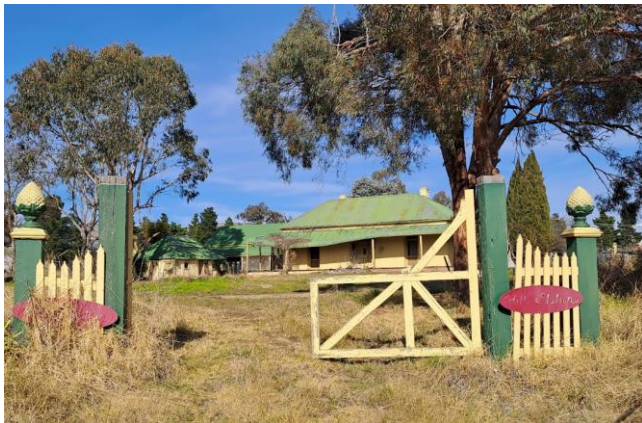
Photo 6.3 View of the dilapidated Hill Station cottage, Sheppard Street
