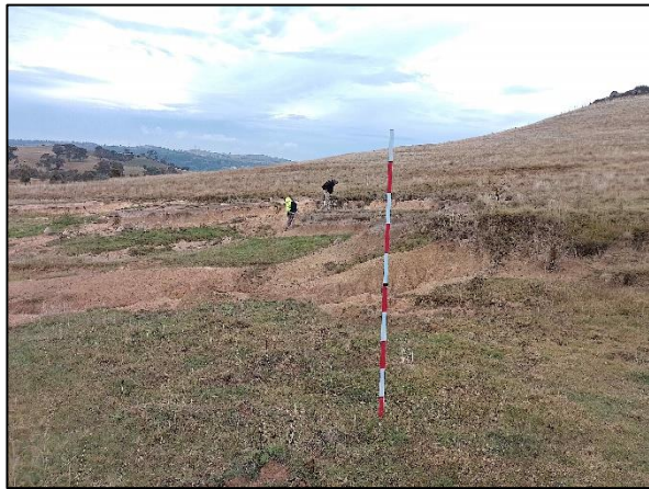
Plate 7. Several drainage line confluences meet in an area of large exposures with heavy erosion. Area between transmission towers 221A and 222A.
