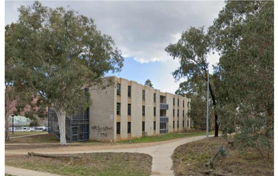
The dilapidated buildings on site in 2018, seen from Aikman Drive (Google, 2025)
