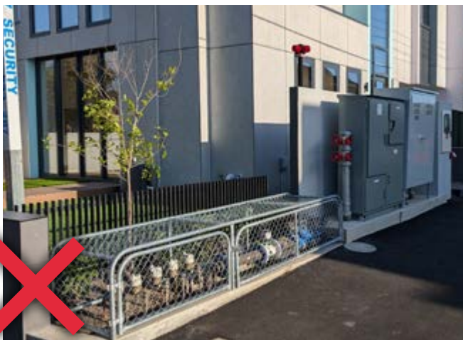
Photo 47: Consolidating services infrastructure to the street without any landscaping or architectural screening reduces the visual amenity and can be dangerous to the general public.
